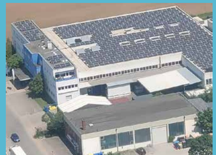
Photovoltaic system on the roof of the TRAMAG building
